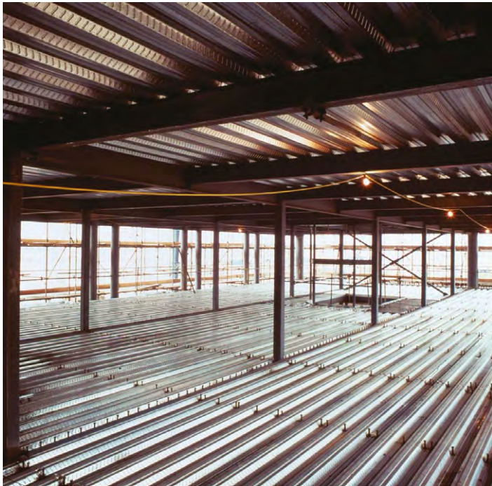
Figure 2: A continuous floor plate awaiting concrete pouring. Rows of studs indicate the beam lines, and even with continuous concrete the slabs will be designed to be simply supported at these points (at ambient temperature)
